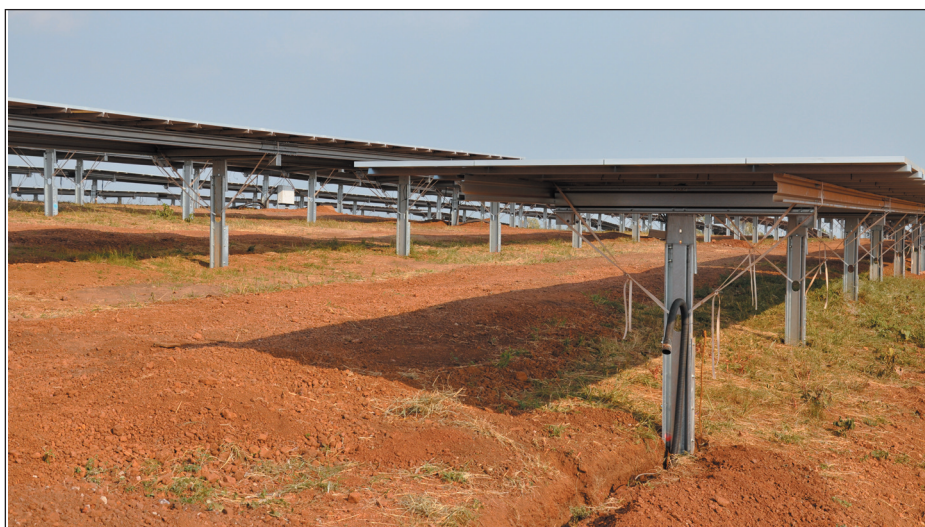
Solar PV panels installed at Gigawatt Global Project
