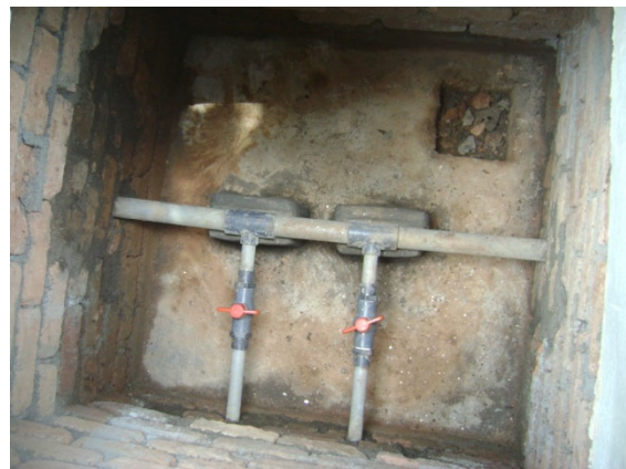
Control valves box 2
