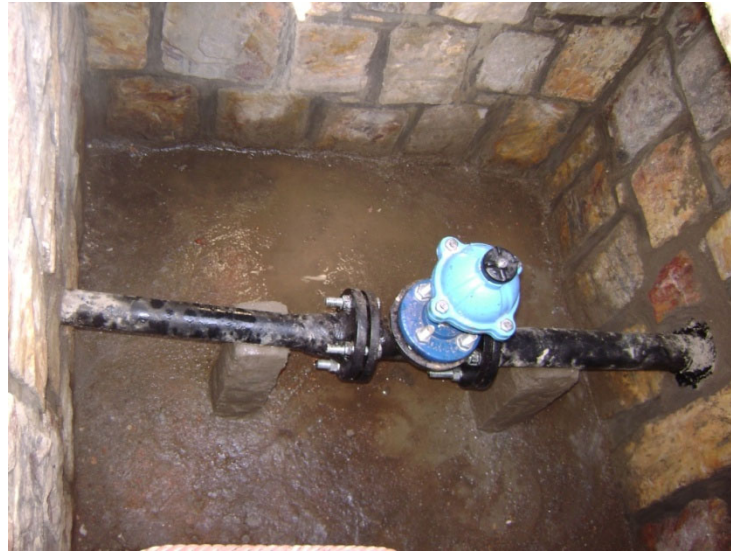
Figure 17: Picture of an air release valve
