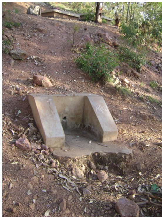
Figure 18: Soak away / tail end of a washout
