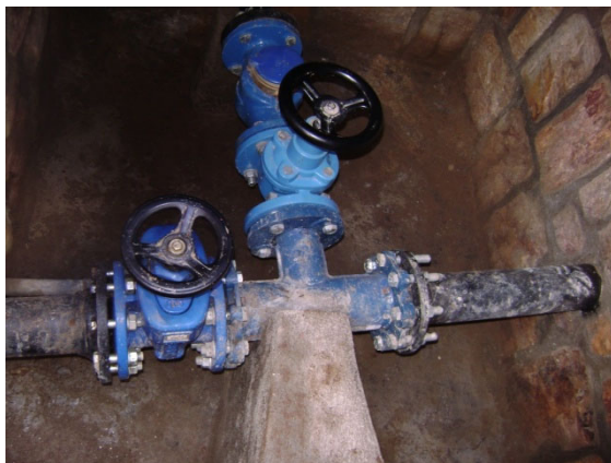
Control valves box 1
