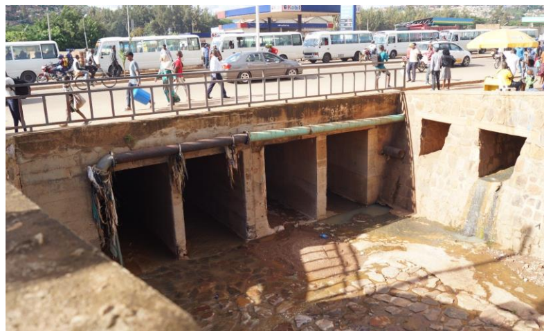
FIGURE 11. NYABUGOGO TRANSPORT HUB BRIDGE ON MPAZI CHANNELIZED RIVER THAT IS PERIODICALLY DAMAGED BY FLUSH FLOODING
