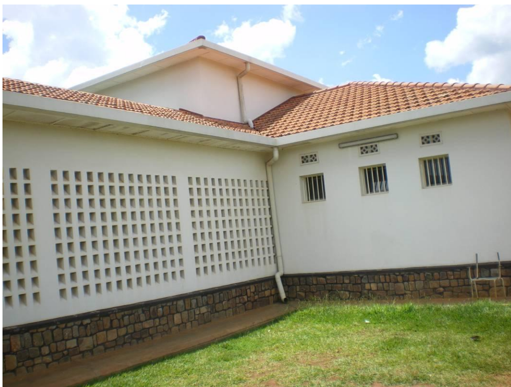
Picture 1.1: Building with partial rainwater collection system – Rainwater is collected but conveyed into drainage channel without being used
