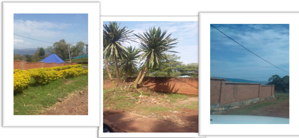
The three boundary walls that will be partially damaged during the construction of the roads
